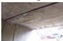
2 - Platta - Armeringsstål - Korrosion 2010-04-27
