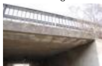
2 - Platta - Armeringsstål - Korrosion 2010-04-27
