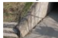
3 - Vingmur - Armeringsstål - Korrosion 2010-04-27
