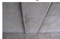
2 - Platta - Armeringsstål - Korrosion 2010-04-27
