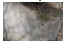
3 - Vingmur - Armeringsstål - Korrosion 2010-04-27
