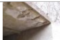
2 - Platta - Armeringsstål - Korrosion 2010-04-27
