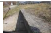
2 - Platta - Armeringsstål - Korrosion 2010-04-27
